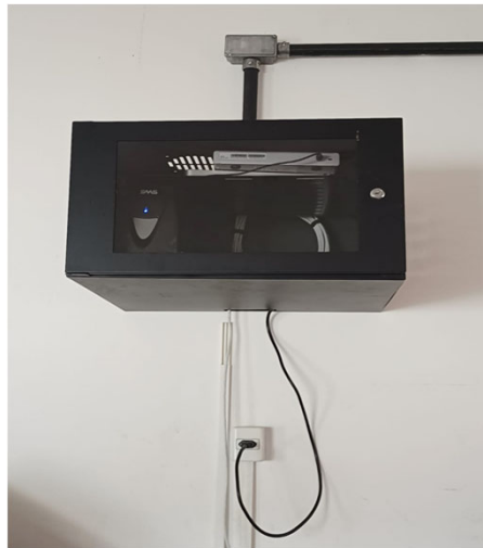
Firewall, Switch e Nobreak
